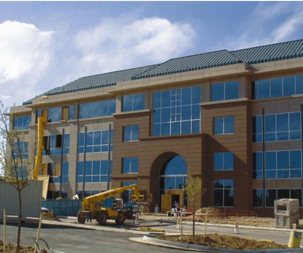
The buildings are designed to provide a corporate identity — and to be marketable in case CH2M Hill ever moves or downsizes.
